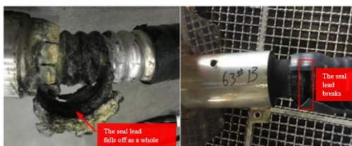
Figure 10: Failures in High-Voltage Cable Lead Seals
