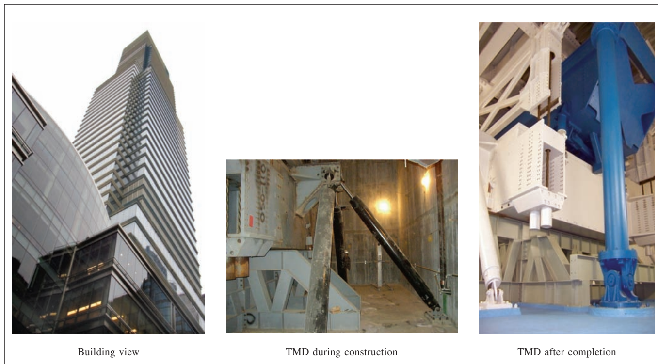
Fig. 8. The articulated mass TMD system installed in Bloomberg Tower in New York City.
